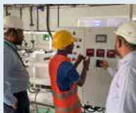
Operation and Maintenance Services
